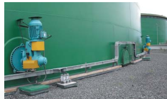
55kW Swivel Gear Mixers installed with Automatic Actuator
